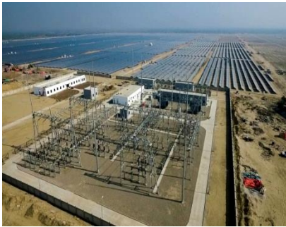
Quaid e Azam Solar Park Project
