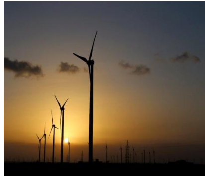
Jampir Wind Power Plant
